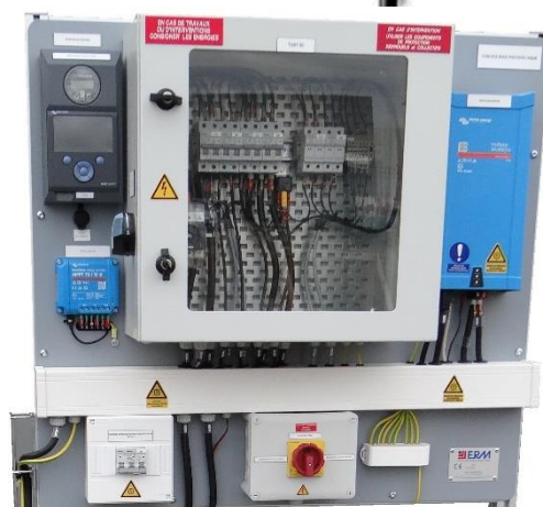
Control panel with switch cabinet
